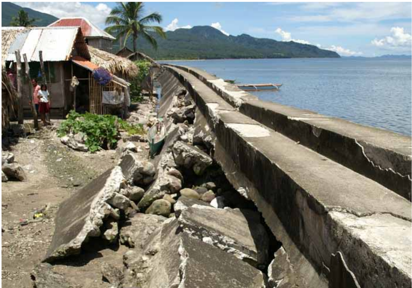
Damaged sea wall, Sorsogon City. © UN-HABITAT / Bernhard Barth
